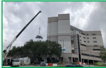
Mechanical Infrastructure Projects
